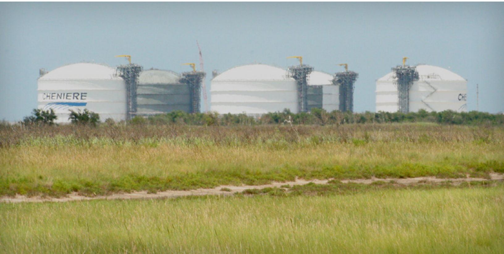
Five storage tanks at the Sabine Pass regasification facility (under construction). June 13, 2009. (Flickr user Roy Luck, CC license BY 2.0)
